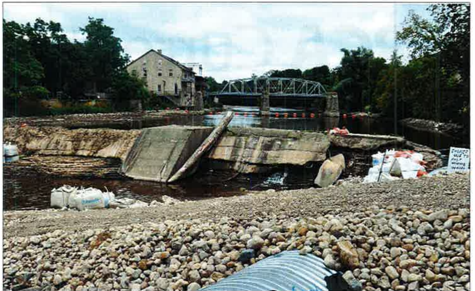
Construction is underway on the Drimmie Dam in Elora and during construction photos of the progress will be posted on the GRCA's Facebook page.
