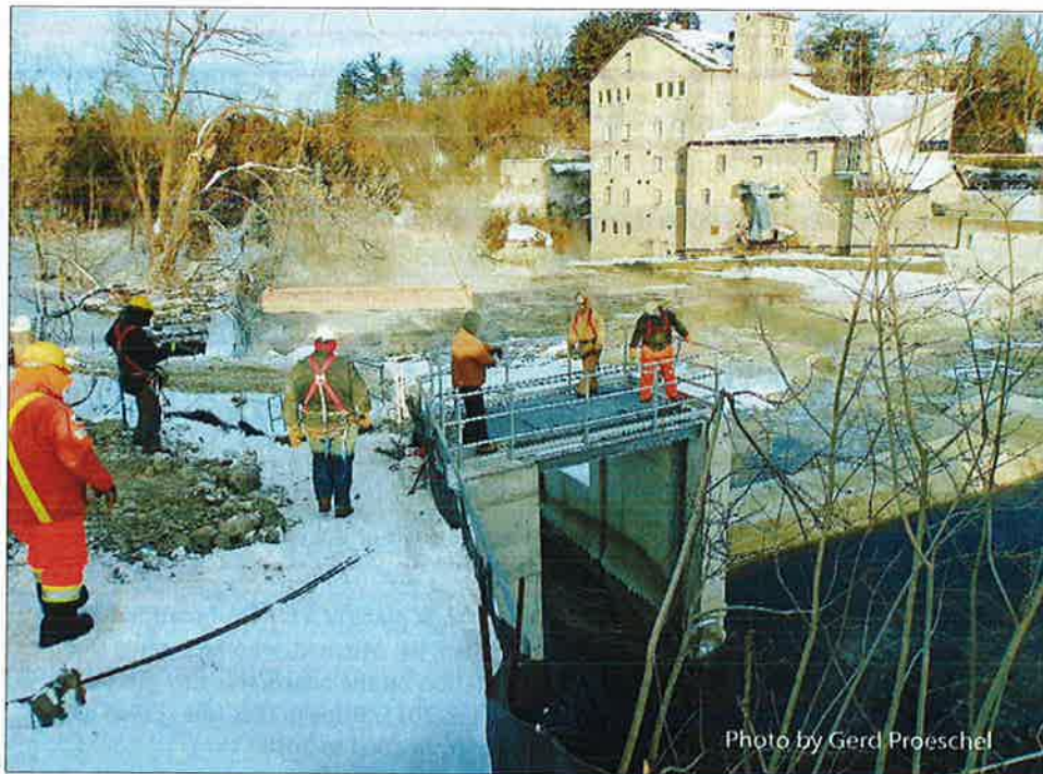
The stop logs were put in place on the new Drimmie Dam in Elora in January on a very cold day. Construction has been underway throughout the winter.
