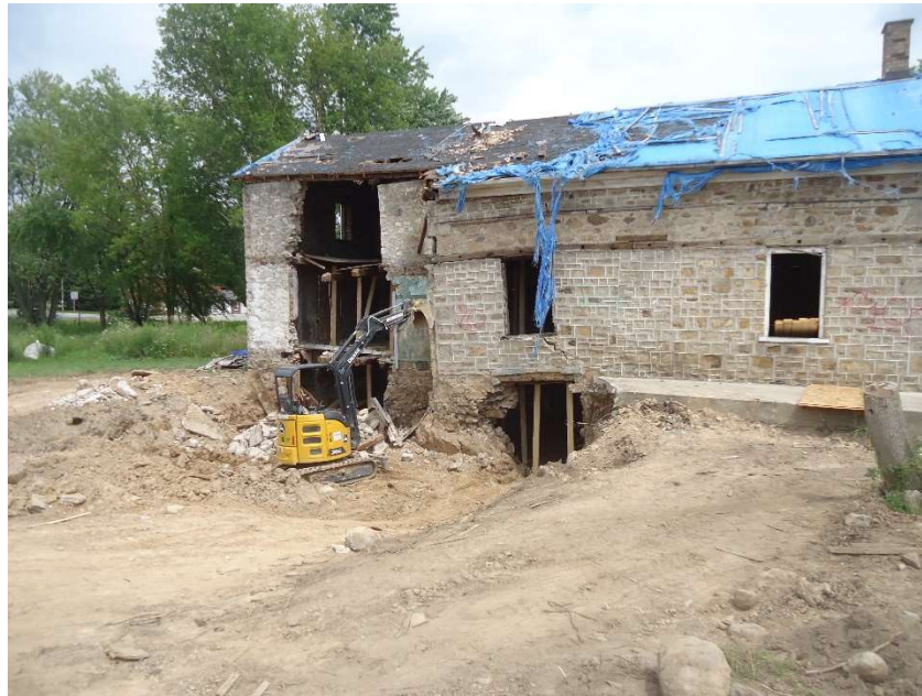
Photo 4: Wall appears to have a significant lean to the left of the second floor window opening. The foundation wall below this section appears unstable. Also note holes in the roof and no windows will allow moisture to continue to enter the building and damage the structural framing.
