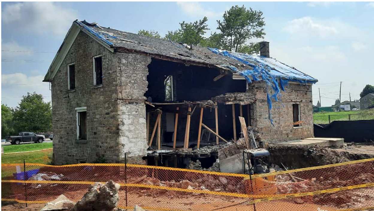
Figure 2 CBO Photo of collapsed wall taken August 11, 2021 after rainfall on August 10, 2021.
