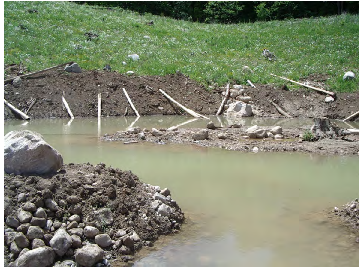
Photo 8 – View of Wetland SW1 immediately after construction. Larger rocks and logs were used to create habitat features. GEC 2022-06-10
