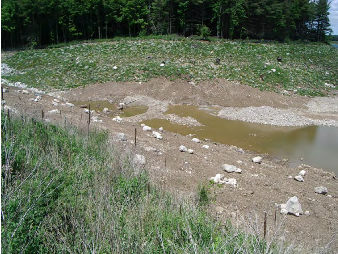
FP05cx - View looking west northwest towards Woodland Protection Zone 'B' and Unit RSW2. Panorama - Left - GEC 2022-06-10
