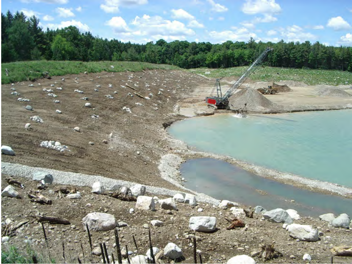
Photo 1 – View looking west along Rehab Slope RSW3. Newly-created Wetland SW3 is in the lower right. GEC 2022-06-10
