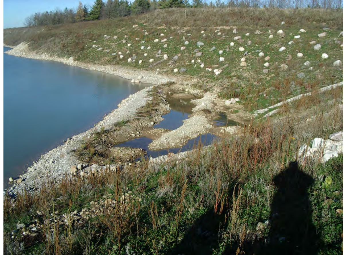
Photo 6 – View looking northeast towards Rehab Slopes RSW4 and RSM2. Wetland SW3 is in the centre of the photo; note the seasonal decline in water level, relative to June (see Photos 1 and 2). GEC 2022-11-09
