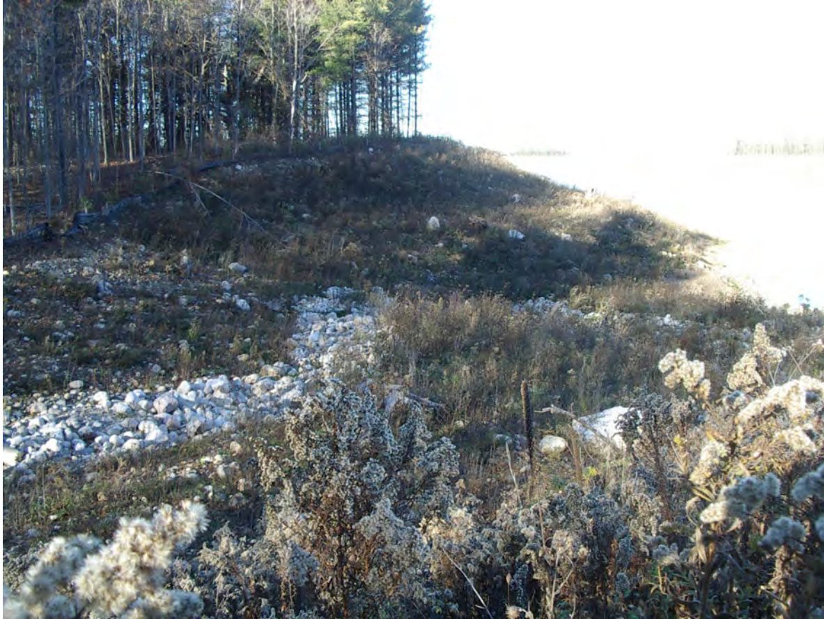
FP03b – View looking north towards Woodland Protection Zone 'B' and Unit RSW1. GEC 2022-11-09
