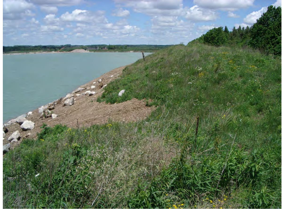
FP10a - View looking north along Unit EB1 and towards Unit EB2. GEC 2022-06-10
