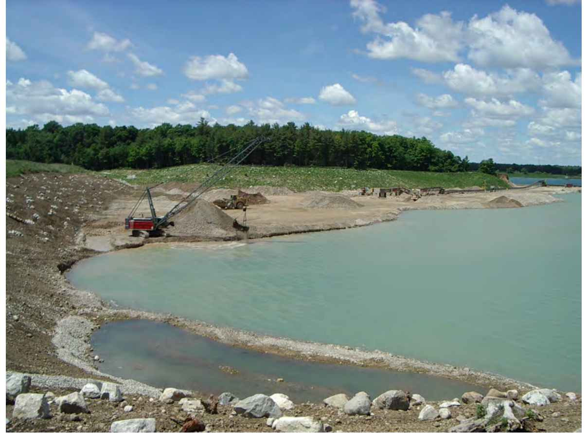
Photo 2 – View looking west northwest towards Rehab Slopes RSW1 and RSW2. Below water table extraction continues, as the Phase 2/6 Lake expands in size. GEC 2022-06-10
