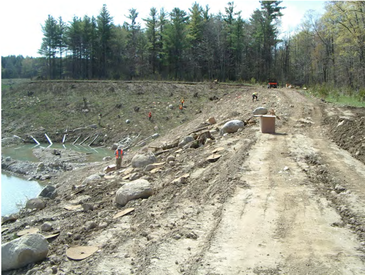
Photo 7: View looking south at side slope Unit RSW1 and Shoreline Wetland SW1. GEC 2023-04-27
