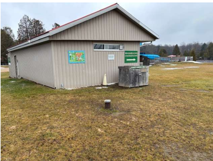
Figure 6 Supply well for field washrooms at water park and concession stand
