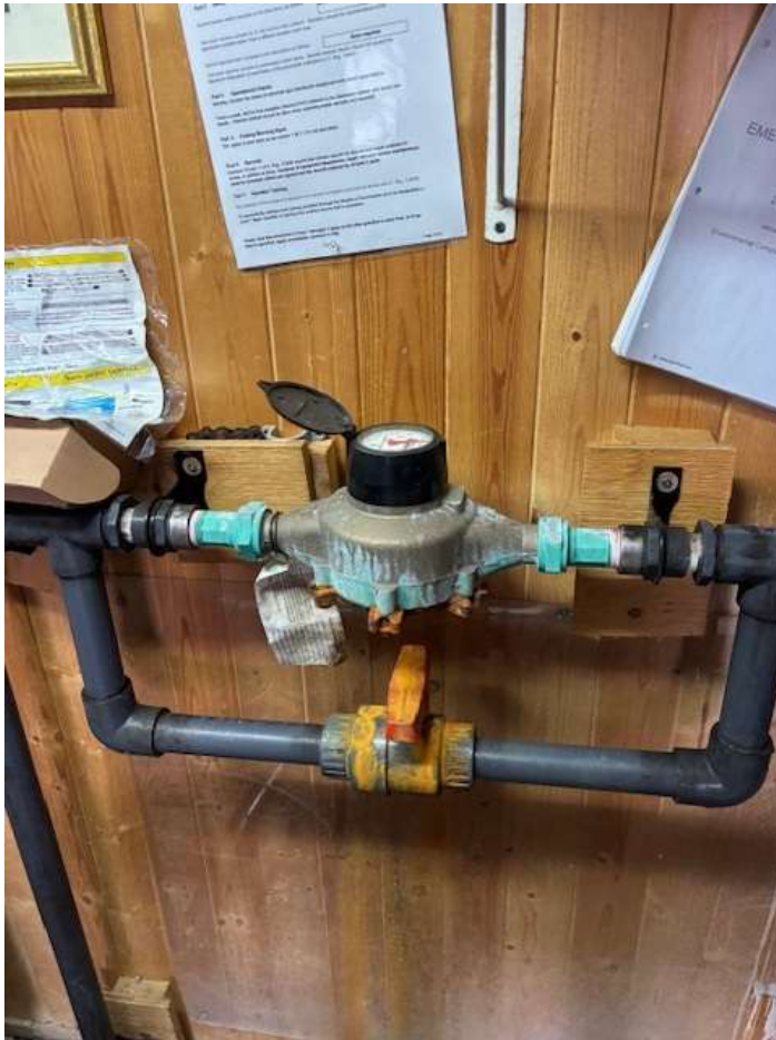
Figure 12 Water meter for distribution water flow, office WTS
