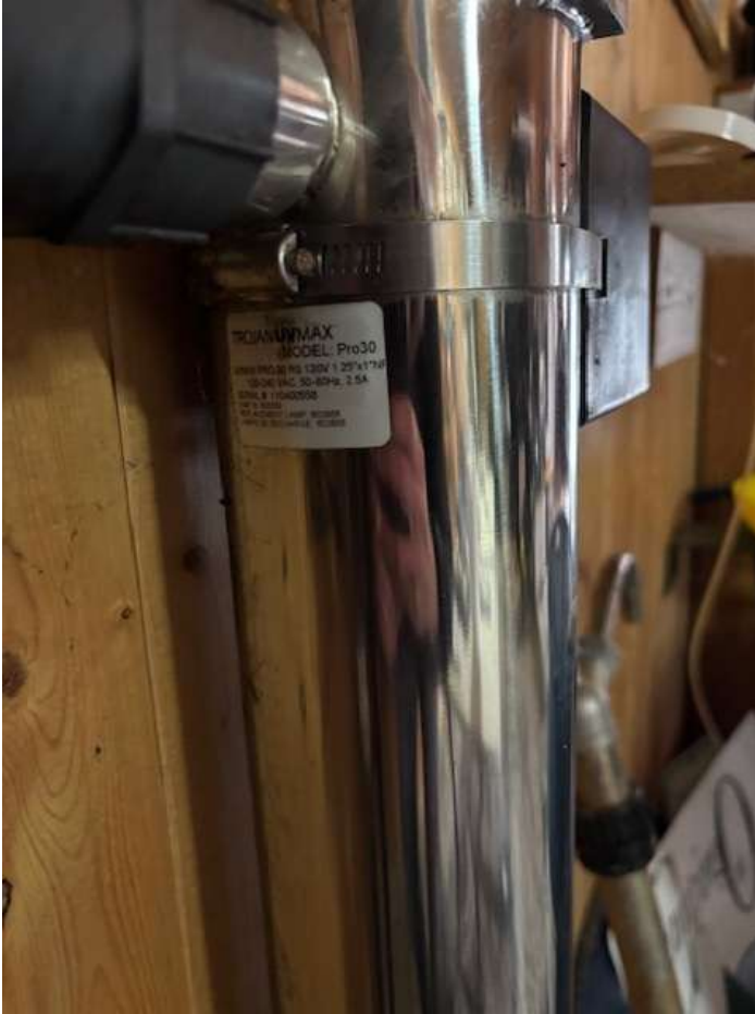
Figure 10 UV disinfection reactor in office WTS
