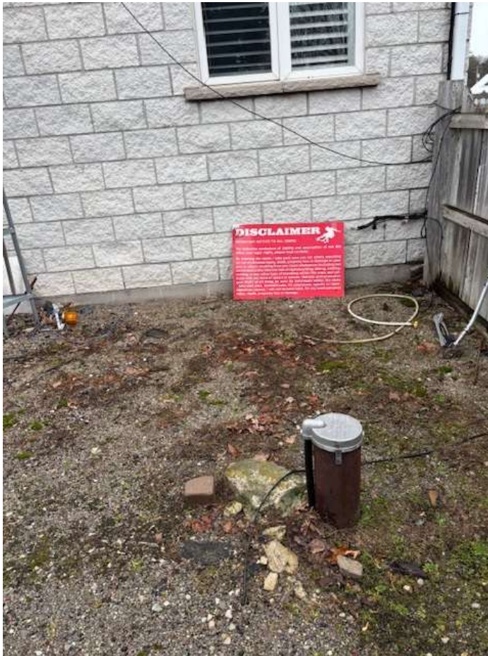
Figure 7 Supply well for WTS in office building
