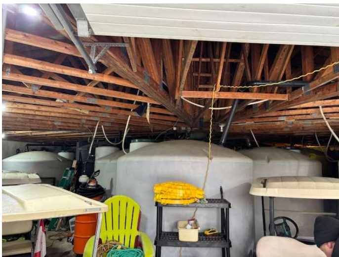
Figure 17 WBF process media tanks in treatment building.
