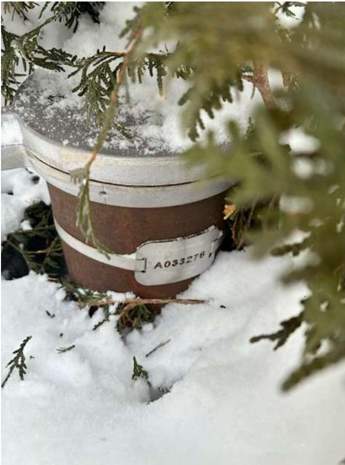
Figure 4 Well for banquet hall WTS
