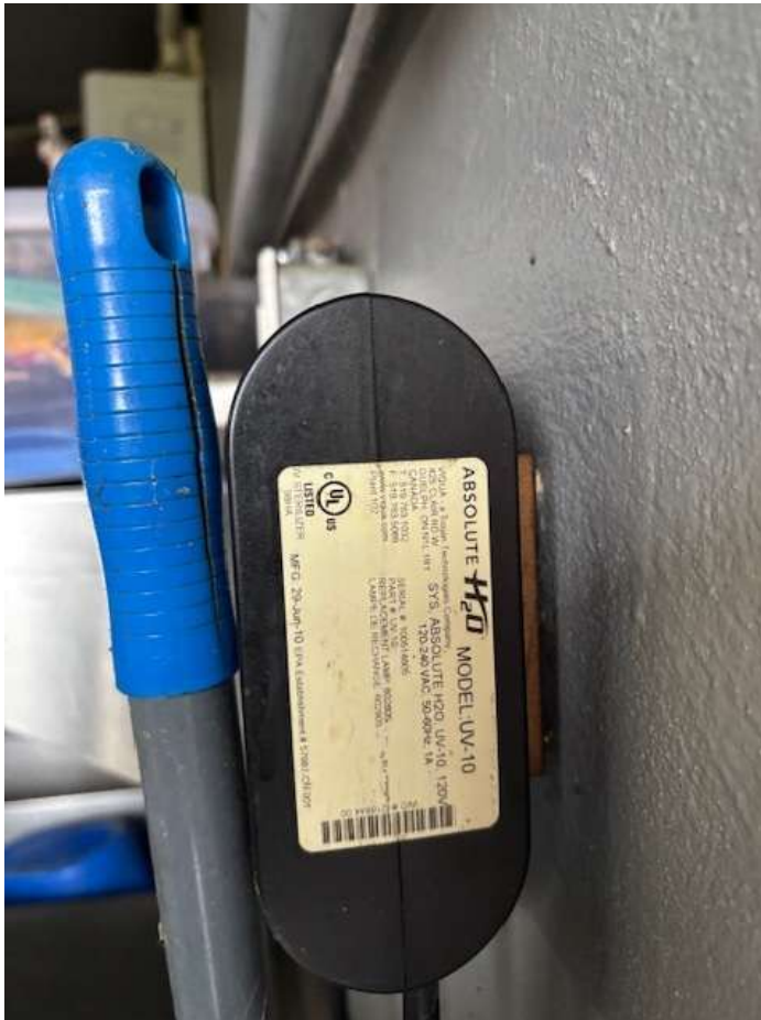
Figure 9 POE UV disinfection reactor information panel
