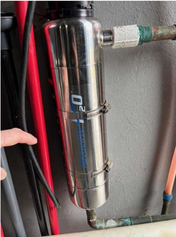
Figure 8 POE UV disinfection reactor, water park concession stand
