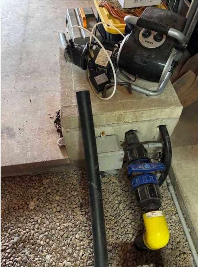
Figure 11 Chlorine pump and reservoir riser with cover, office WTS
